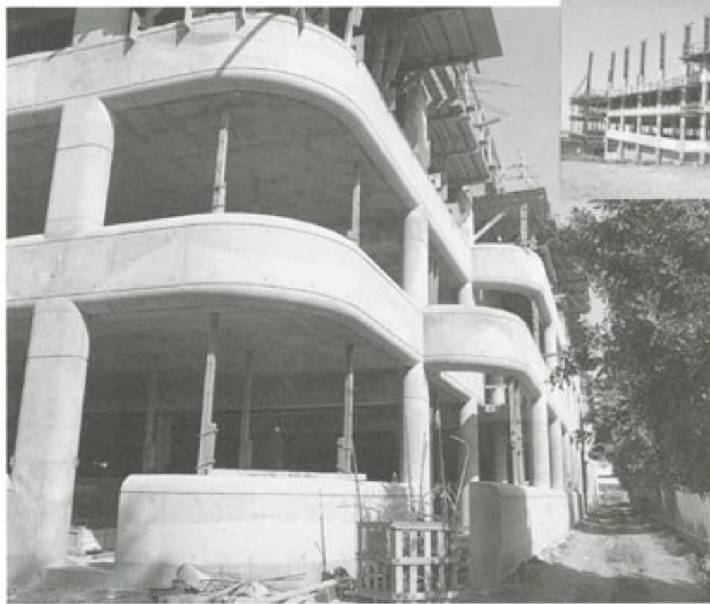
When completed in April of '92, the Visitor Paid Garage at the Santa Clara County Government Center in San Jose, California will have five levels, housing over 420,000 sq. ft. of space.
